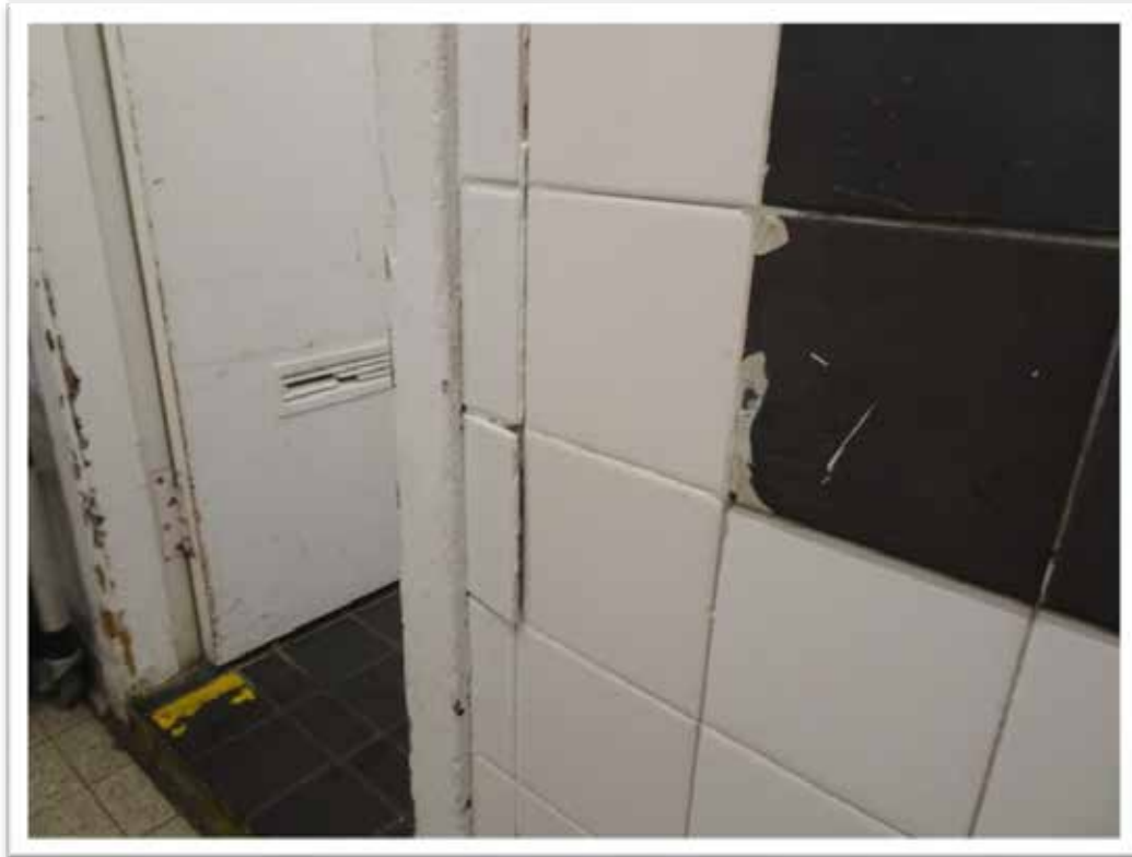
Unclean tiles in kitchen
